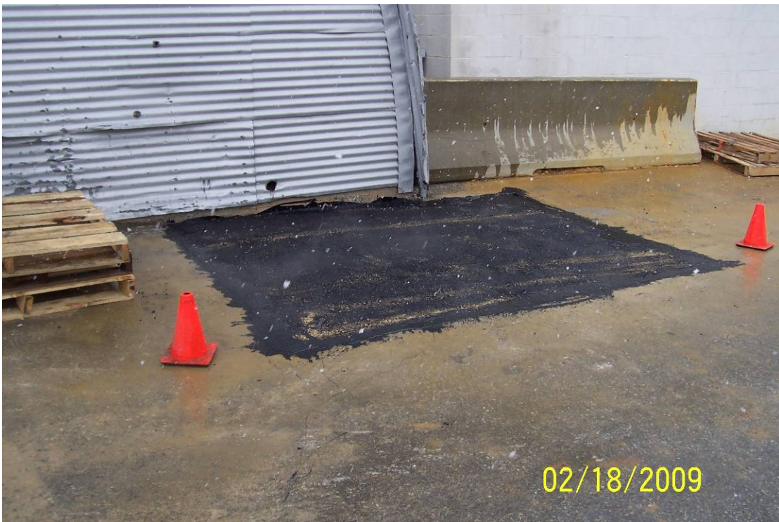
Photo 10- View of Pit#2 and sump outside Building 51 finished to grade with asphalt. View facing northeast.
