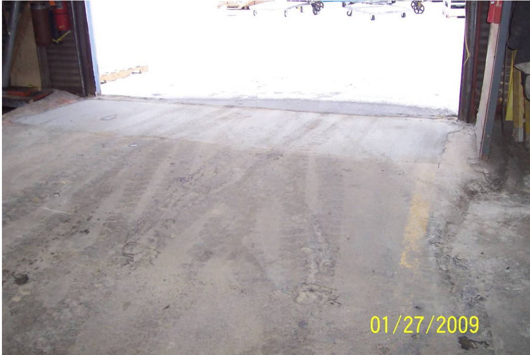
Photo 17- View of entrance slab to Building 51 completed to grade with concrete. View facing south.
