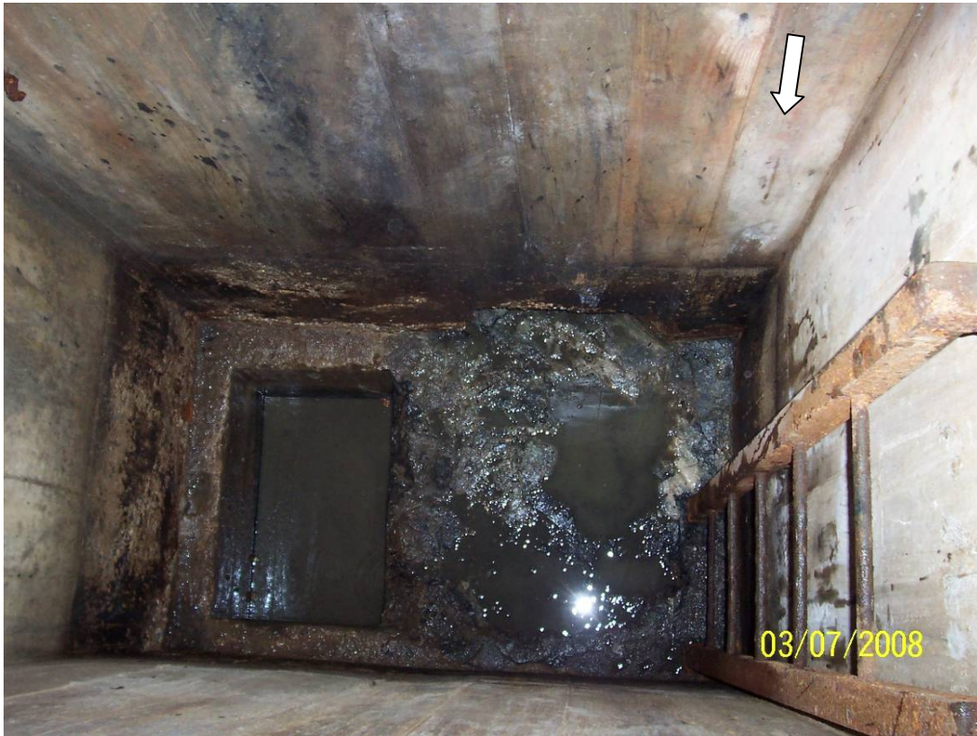
Photo 3-View of Pit#1 and sump inside Building 51 after pipe removal. Sludge was removed prior to closure. North indicated by white arrow.
