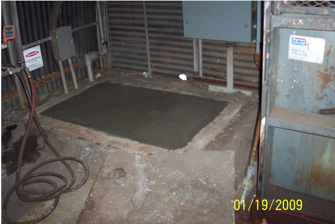
Photo 5-View of Pit#1 and sump inside Building 51 finished to grade with concrete. View facing southeast.
