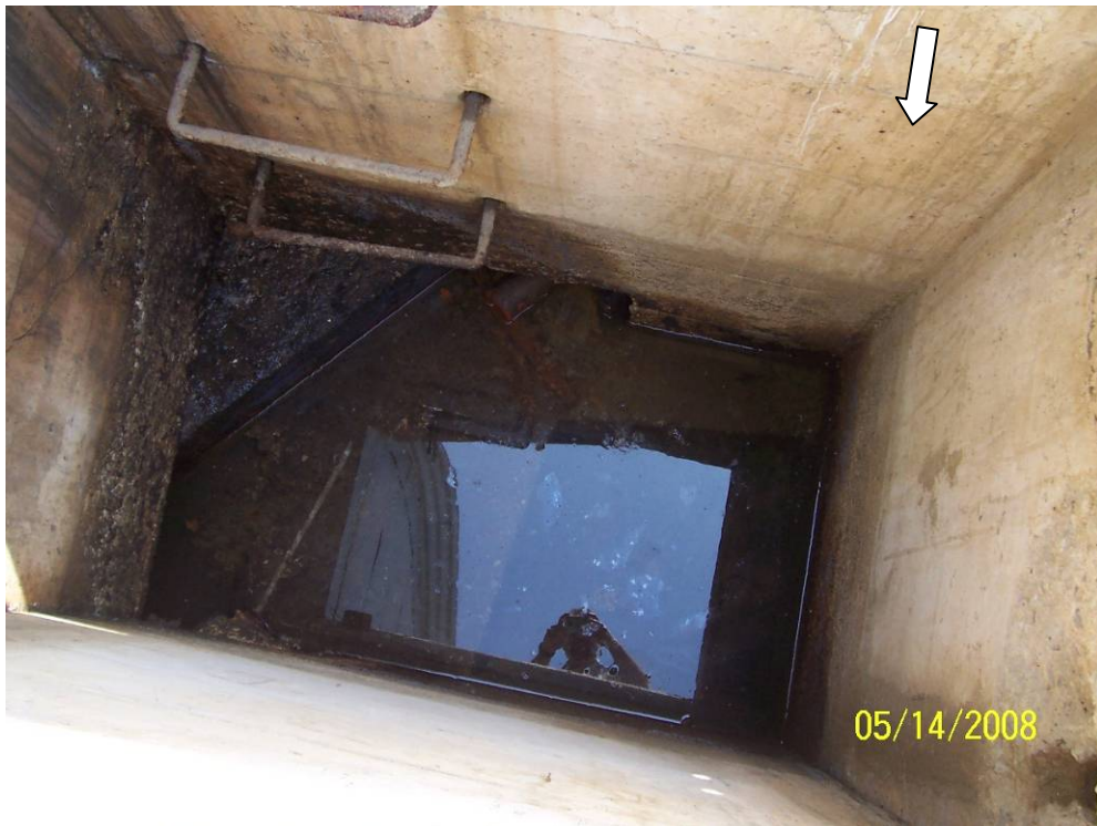
Photo 8- View of Pit#2 and sump outside Building 51 after cleaning and pipe removal (note rainwater has partially filled pit). North indicated by white arrow.
