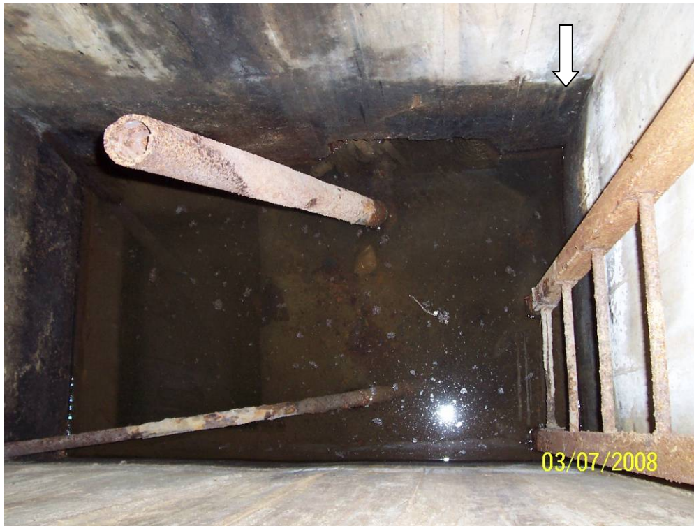
Photo 2-View of Pit#1 and sump inside Building 51 prior to cleaning and pipe removal. North indicated by white arrow.
