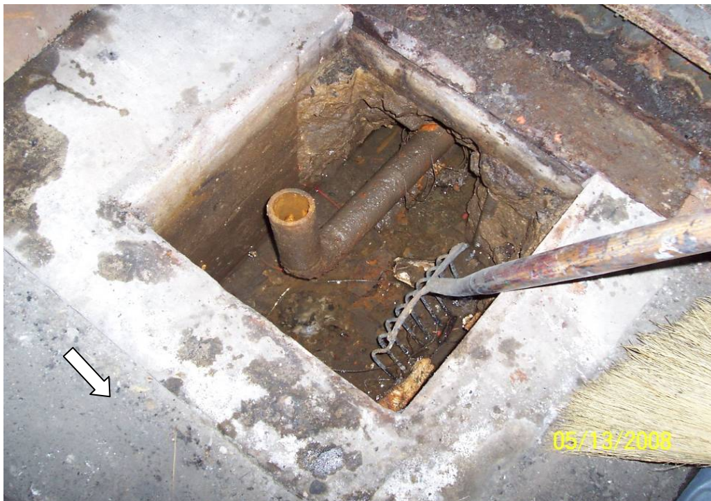
Photo 12 – View of Pit#3 during cleaning and prior to pipe removal. North indicated by white arrow.
