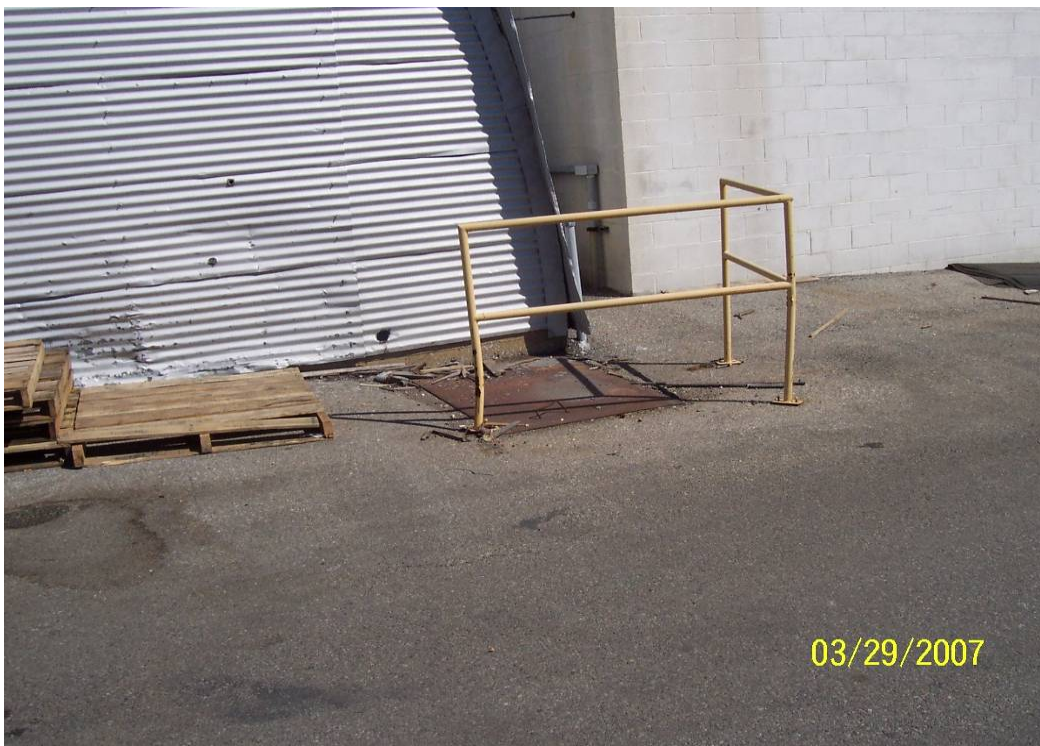
Photo 6 – View of Pit #2 at exterior southeast corner of Building 51. View facing north.
