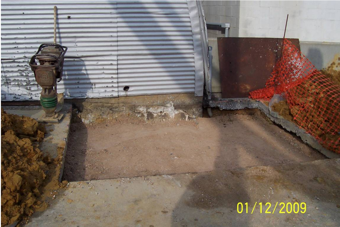
Photo 9- View of Pit#2 and sump outside Building 51 after backfilling. View facing north.
