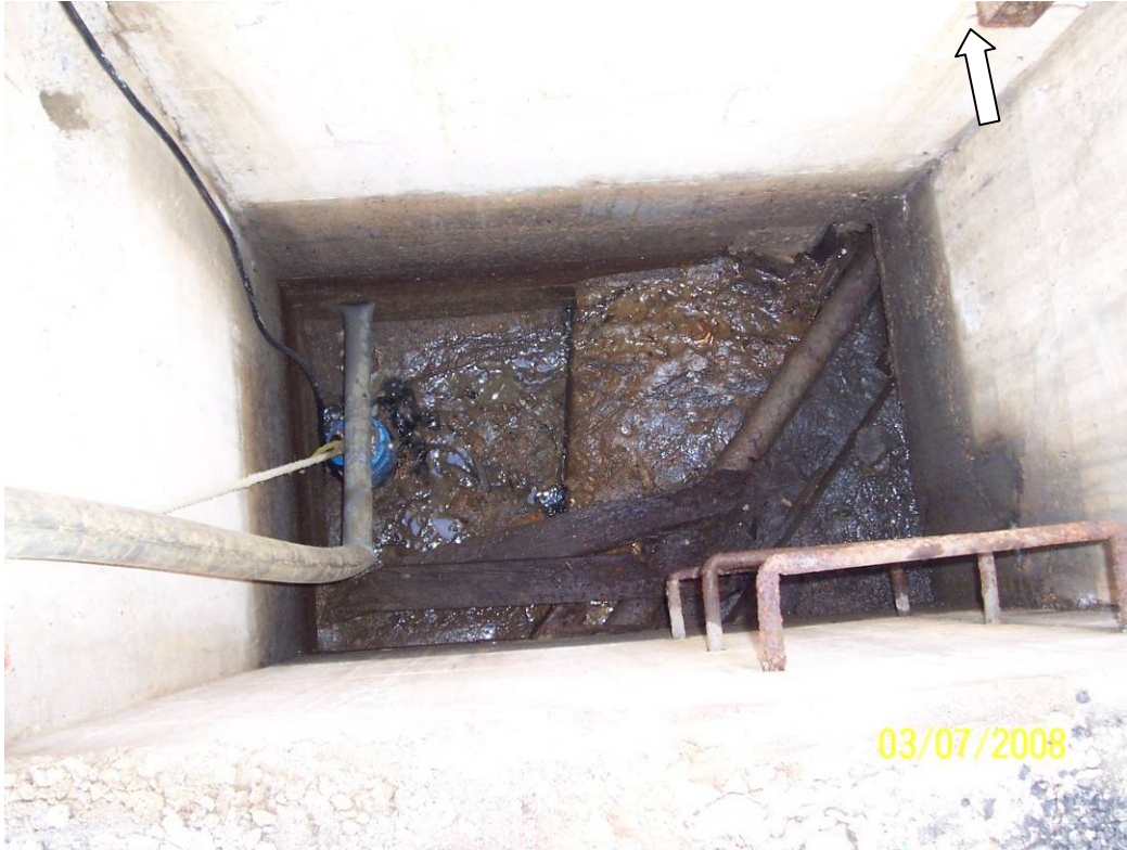
Photo 7-View of Pit#2 and sump outside Building 51 prior to cleaning and pipe removal. North indicated by white arrow.
