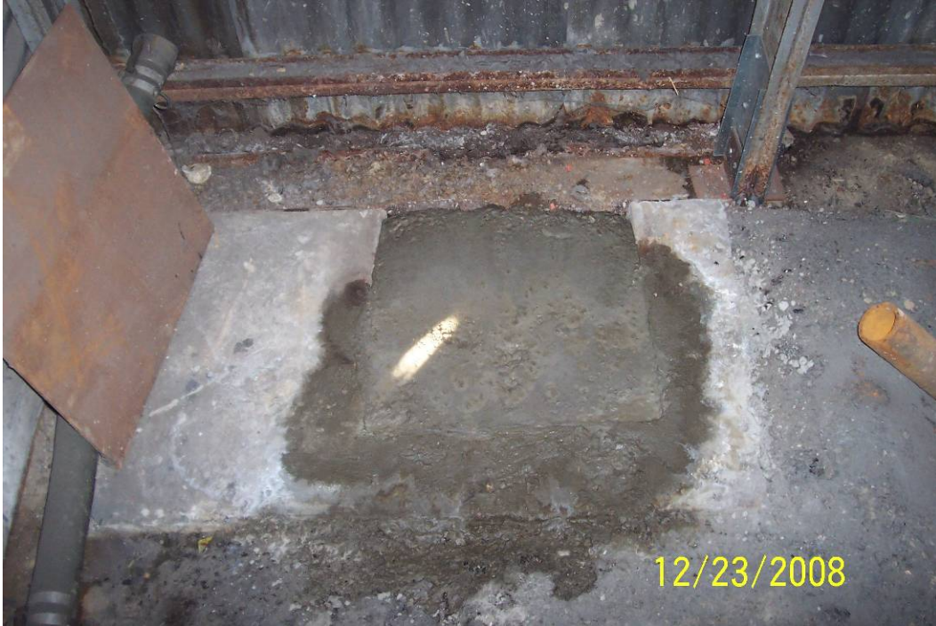
Photo 13- View of Pit#3 inside Building 51 finished to grade with concrete. View facing west.
