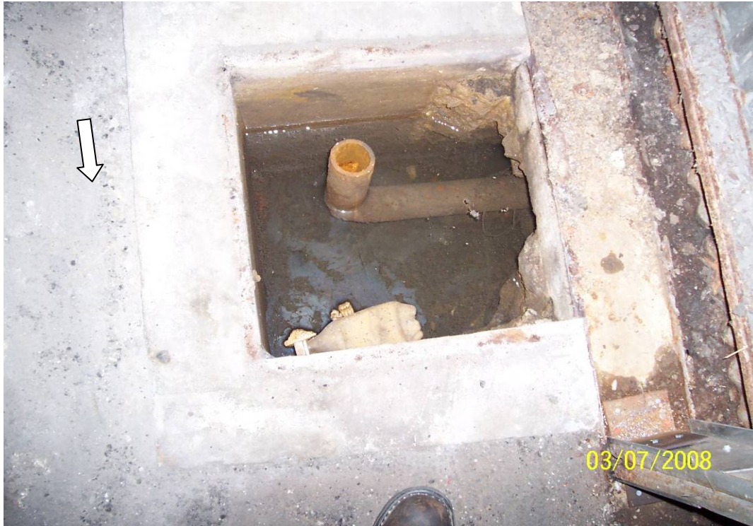
Photo 11- View of Pit#3 inside Building 51 prior to cleaning and pipe removal. North indicated by white arrow.
